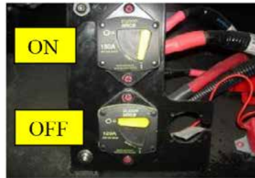
Breakers at rear of coach
