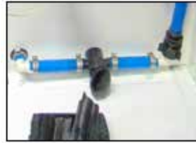
Water supply shutoff to the cartridge water filter (shown OFF)
