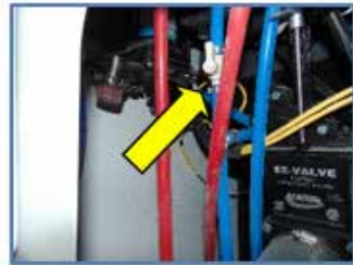
Pump Backflow Valve
